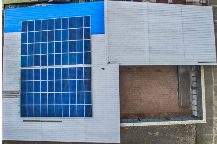
Fig. 1. Photovoltaic system of 20 kW installed in Andagoya - Chocó, Colombia.
