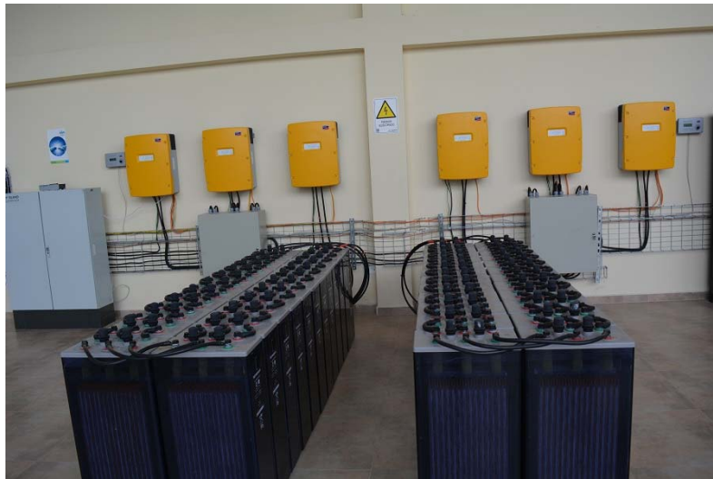
Fig. 2. Installed battery bank and islanded inverters.
