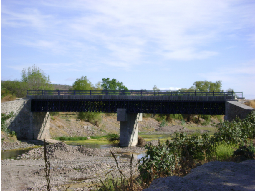
FIGURE 4. Vehicle bridge project completed through 3x1 Program in Atitlan, Jalisco. Photo by author.
