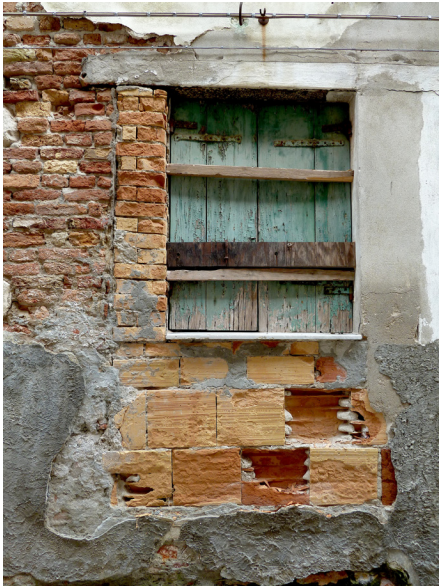
Figure 10.5: Gaps in Venetian brickwork appear to invite visitors to ‘post’ rubbish into the holes that the deterioration has left in the walls, such as this folded wedge of paper, which has been carefully
