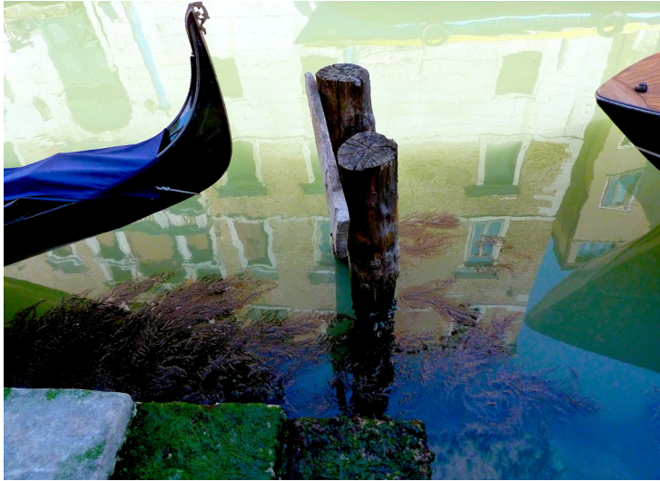
Figure 10.7: The visible wear and tear at this boat mooring's base mirrors the kinds of processes that shape Venice's foundations, which rest upon woodpiles. The salty marine water sank these into the soft delta soil, on which the city was established in mediaeval times, and they have generally been preserved. However, when woodpiles are exposed to the air, they are rapidly digested and transformed by marine organisms, such as bacteria and shellfish, and lose their structural integrity through decay. Photograph, Rachel Armstrong, August 2010.
