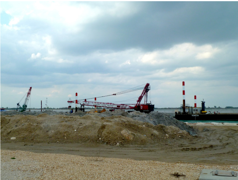
Figure 10.9: Construction site of the MOSE project from the Lido beach. Photograph, Rachel Armstrong, August 2010.
