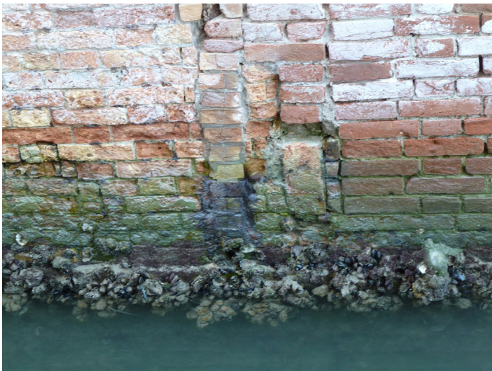
Figure 10.4: Physical processes act in concert with the local organisms like oysters, algae, bacteria and mussels, and produce metabolic events that shape the architectural fabric of Venetian buildings. These entanglements of natural and man-made materials constitute a post-natural building fabric, which functions as a vertical synthetic marine ecology at the tideline. This process may be likened to the production of scar tissue in an organism. Photographs and collage, Rachel Armstrong, August 2010.
