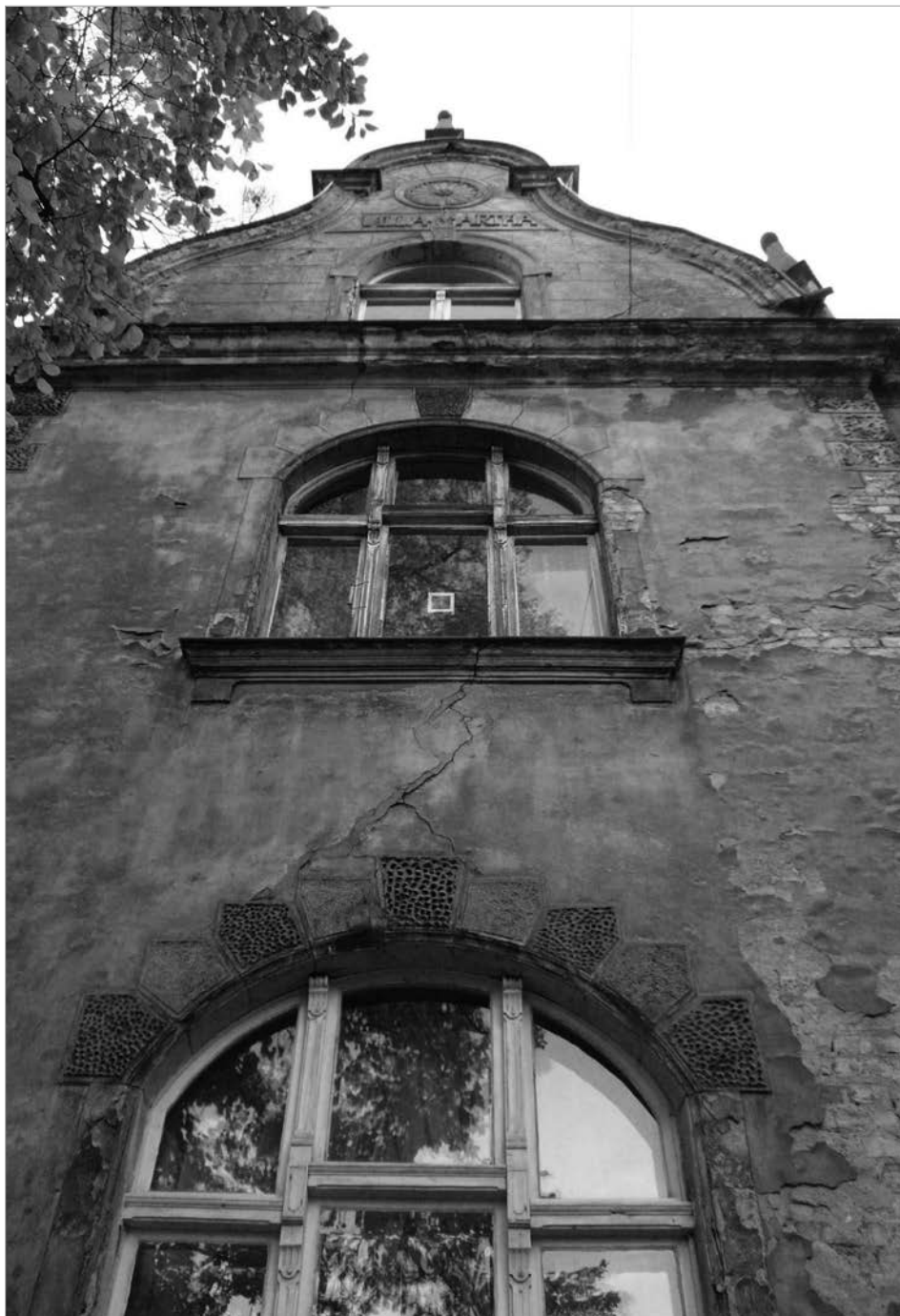
Figure 7. Example of a dilapidated old house in the Oliwa district
